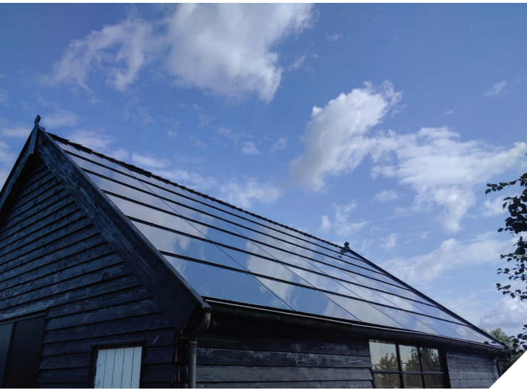
13.05 kWp BAPV system in Sweden
